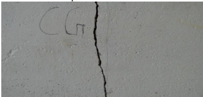
Fig.16 Crack pattern of single layer galvanized panel
