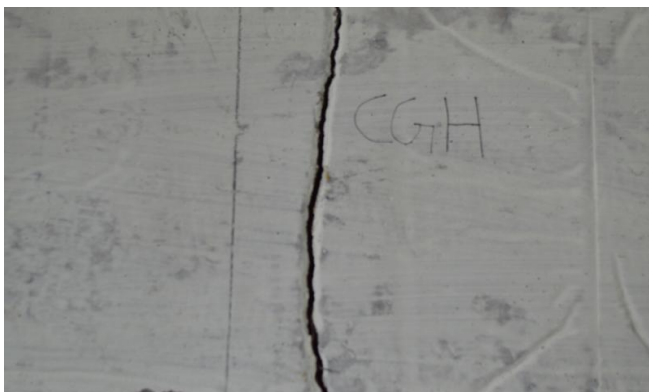
Fig.20 Crack pattern of single layer galvanized panel
