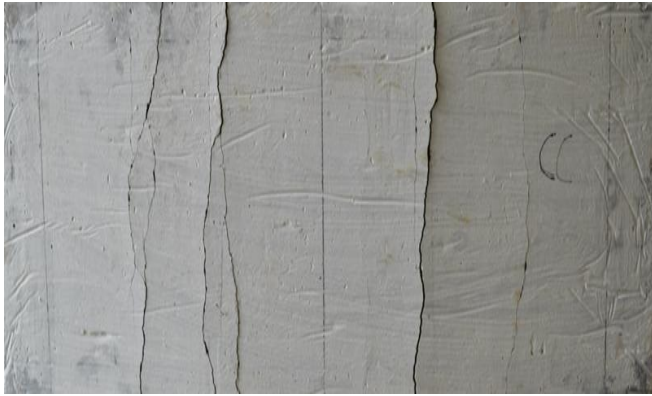
Fig. 24 Crack pattern of single layer crimped panel
