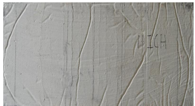
Fig. 29 Crack pattern of 1% inhibited single layer crimped panel
