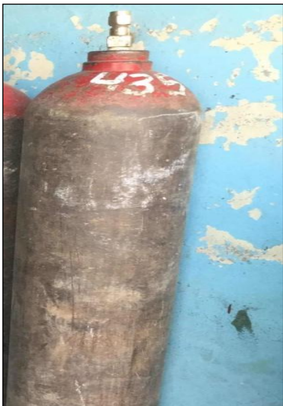
Fig 3. Nitrogen gas cylinder (140 psi pressure)
