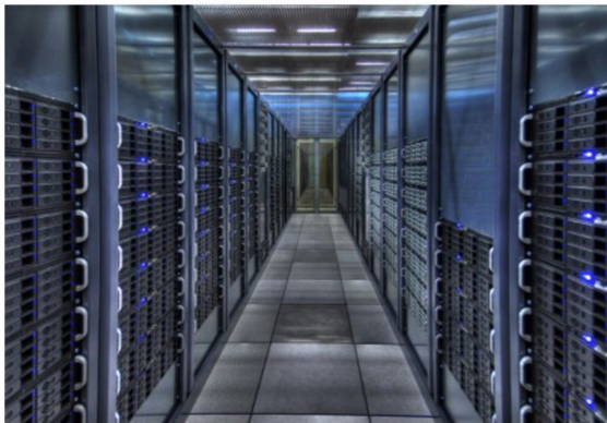
Data storage solutions at the CERN data centre (Image: CERN)
