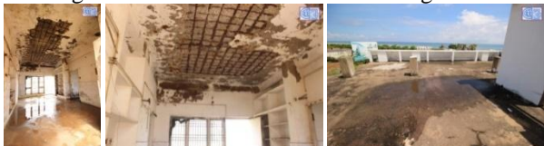
Figure 28 (a) North view (b) Ceiling view (c) Stagnant water on terrace level above the FL 2: Lounge Figure 26 – (CD 04, SD 04, PD 10, 12) GL 2: Toilet – Ceiling view Figure 27 – Terrace level – staircase headroom roof; Figure 28 – (CD 07, SD 07, PD 15) FL 2: Lounge (a) North view (b) Ceiling view (c) Stagnant water on terrace level above the FL 2: Lounge
