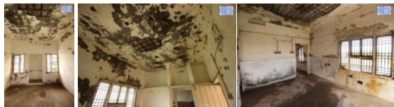
Figure 29 (a) South view (b) Ceiling view Figure 29 – (CD 08, SD 08, PD 26, 28) FL 3: Bedroom (a) South view (b) Ceiling view
