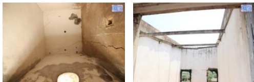
Figure 26 (CD 04, SD 04, PD 10, 12) GL 2: Toilet – Ceiling view Figure 27 Terrace level – staircase headroom roof;
