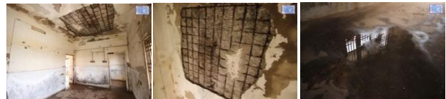
Figure 30 (b) North west view (c) Ceiling view (d) Floor level view showing the movement in water. Figure 30 – (CD 10, SD 09, WD 08, GD 05, PD 18, 19) FL 6: Bedroom (a) North east view (b) North west view (c) Ceiling view (d) Floor level view showing the movement in water.
