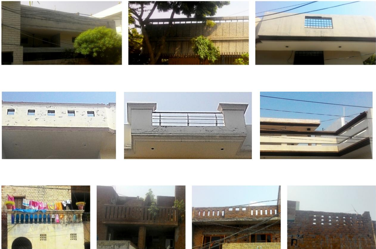
Fig. 4: Images of parapet walls with a range of solid to void ratio along with their design patterns recorded during the visual survey. Source: author
