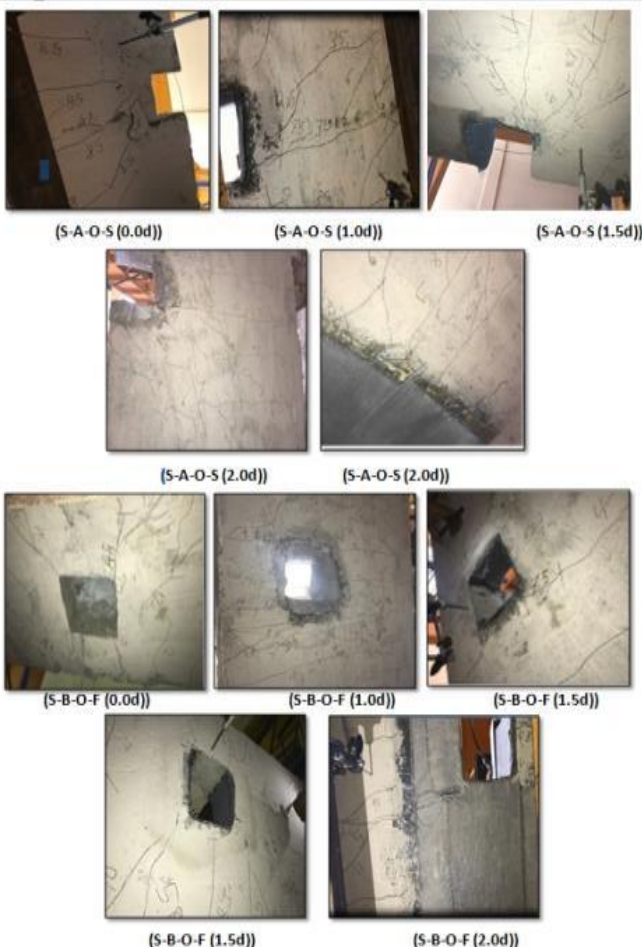
Figure 13. Crack Patterns for Studied Specimens
