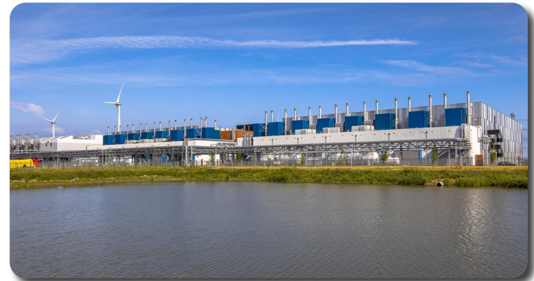
Google's Datacenter in Eemshaven, Netherlands. Access to solar, hydro, and wind energy is increasingly important to minimise the environmental impact of these sites.
