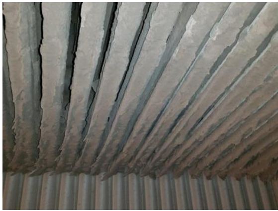
Figure 2: Protective evaporator from below (in the flow direction, luv) after a system operation of 9 weeks
