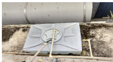
Fig. 8 Water supply form tank
