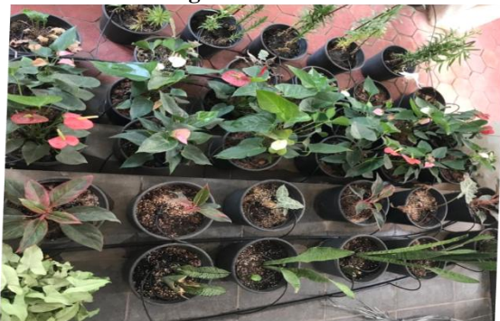
Fig. 5 Drip system installed at patio zone
