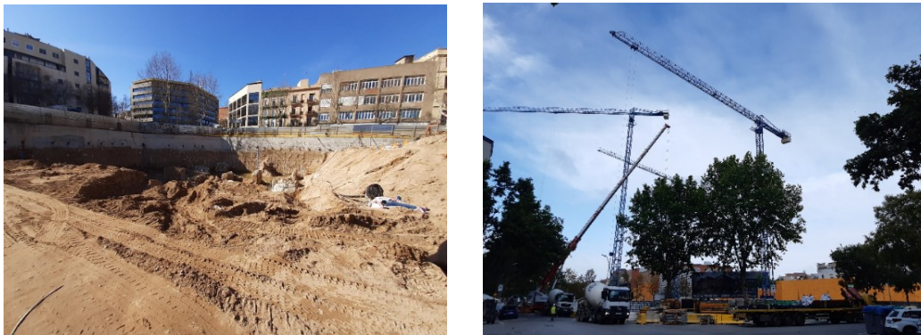
Figure 21: On the left: MILE. Construction site in February 2021 - Excavation levels; on the right construction site in May 2021
