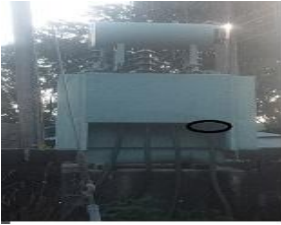
(b) Transformer rating: 500KVA
