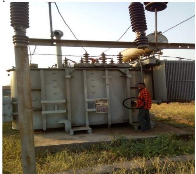
(a) Transformer rating: 7500KVA
