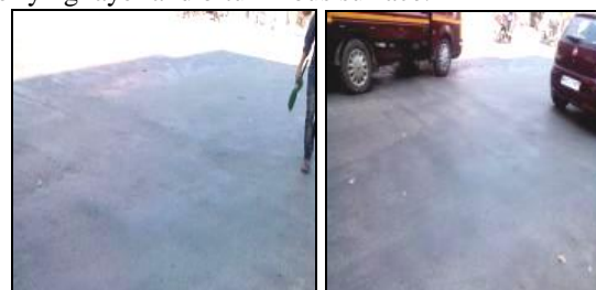
Fig. 14 Bulging of Bituminous Layer
