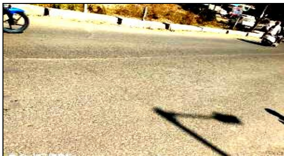
Fig. 23 Bleeding of Bituminous Layer
