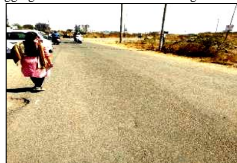
Fig. 22 Bleeding of Bituminous Layer
