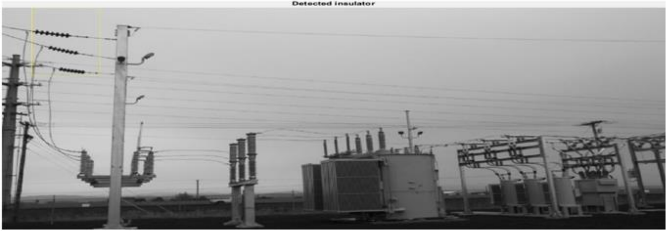
Fig. 13 Location of insulator in a cluttered scene
