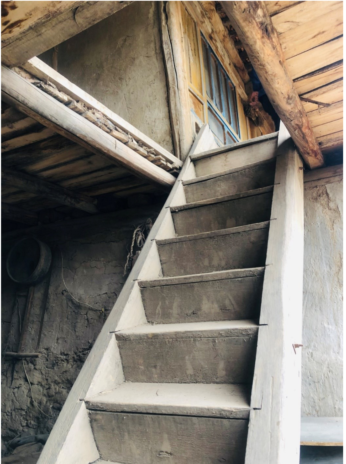
FIG 4. A traditional style old wooden ladder connects the first and second floors (7 June 2020, Jugui).
