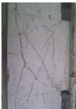
Figure III.13. Cracking pattern in a corner joint under (C. Del Vecchio, M. Di Ludovico, A. Prota and G. Manfredi (2015))
