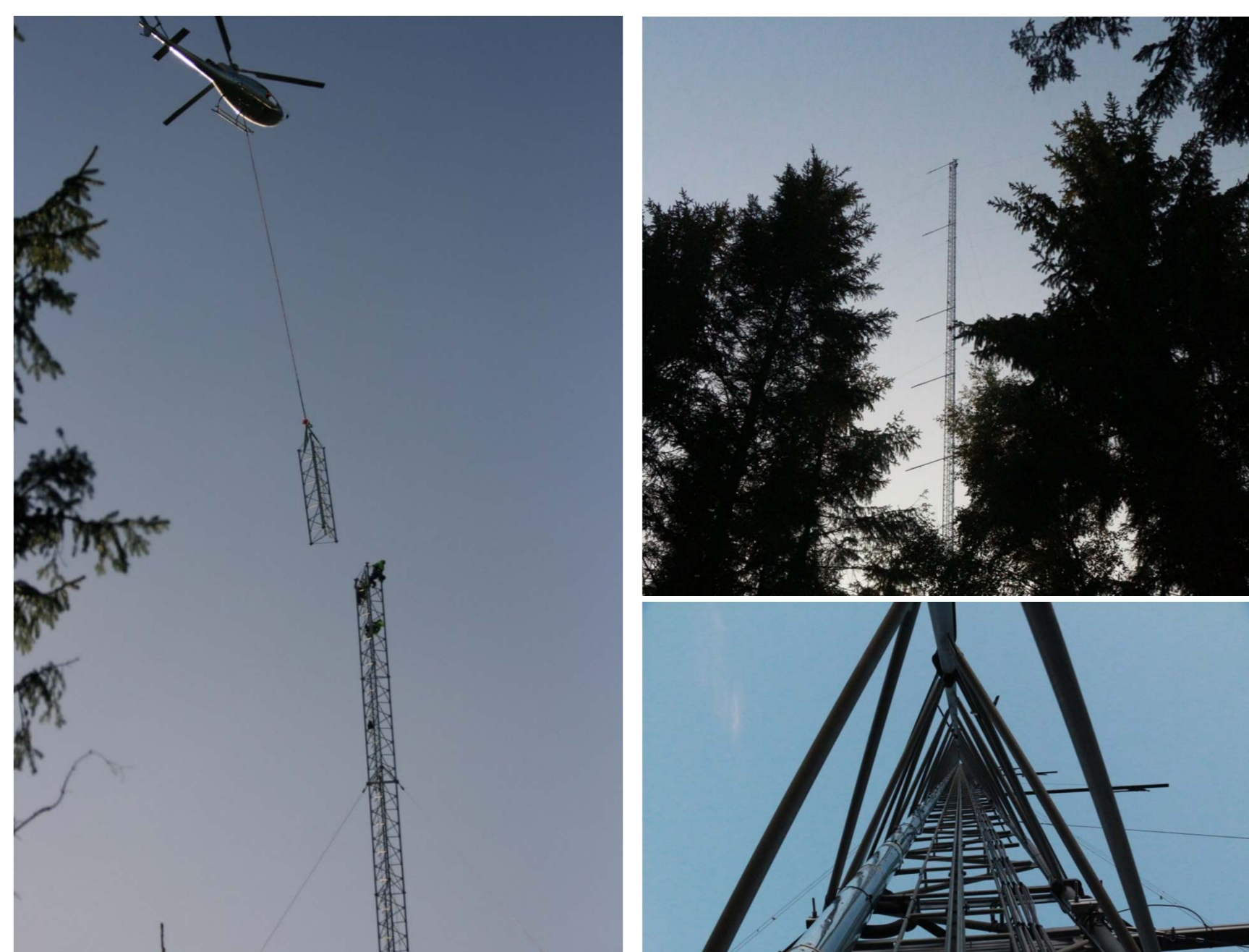
Building the Hyltemossa tower. The tower after being equipped and an inside view
