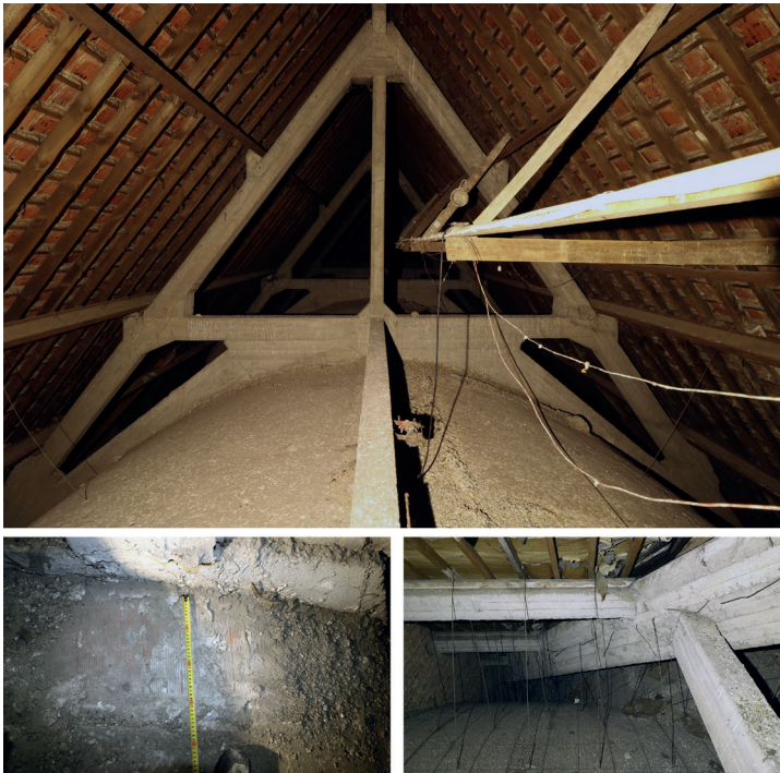
Figure 14. Church of Divin Sauveur; Top: Extrados of the vaults; bottom left: Last bay before the arch of the transept; bottom right: Extrados of the vaults in the transept (Photos: Authors, 2020).
