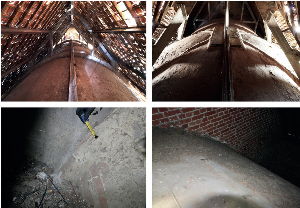
Figure 8. Extrados of the church of Sainte-Alix; Left: Nave; top right: Transept; bottom right: Apse (Photos: Authors, 2019).
