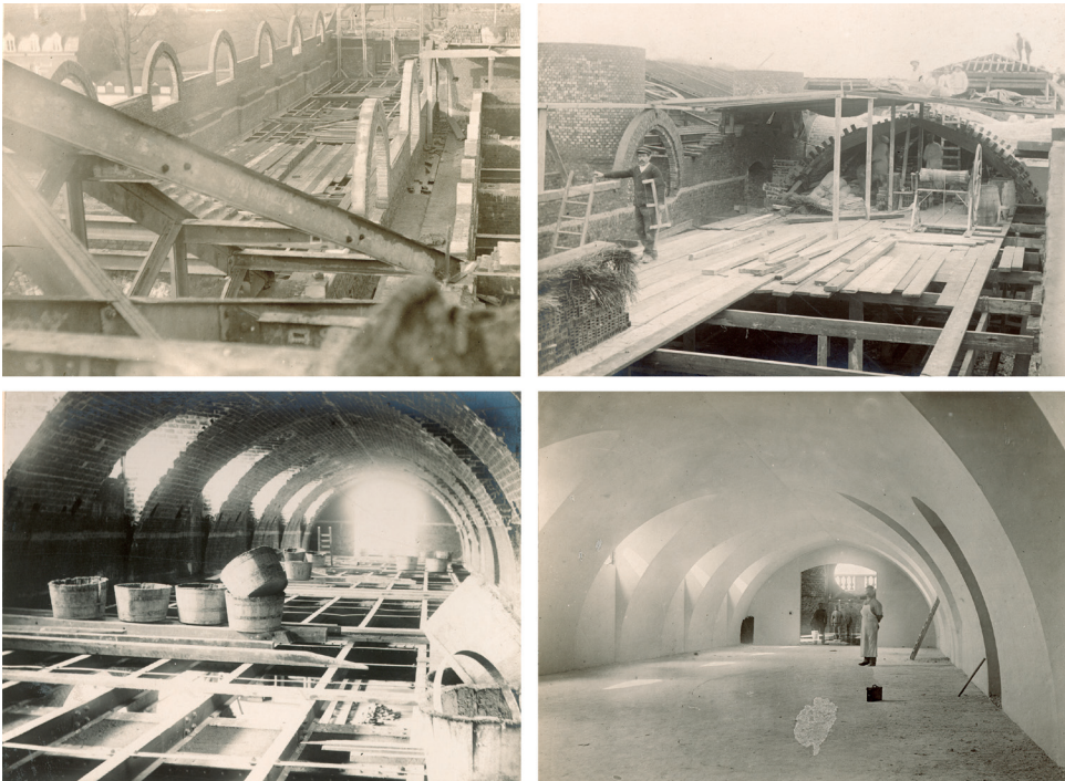
Figure 11. Vaults over the lateral galleries, under construction (HP.1968.10.6–41–44, RMCA Tervuren collection, Charles Girault archives).
