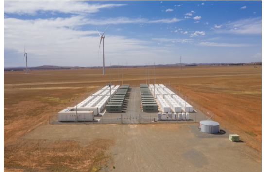
Hornsdale Power Reserve 129 MWh, 100 MW, 56 M€
