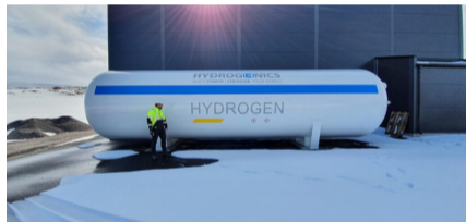
The hydrogen tank outside the containment building
