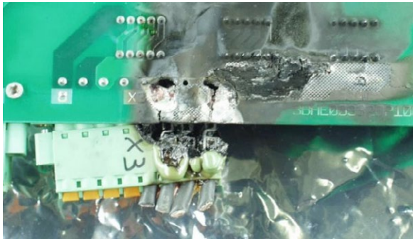
Fig.3 Arcing damage in the PCB at the connector
