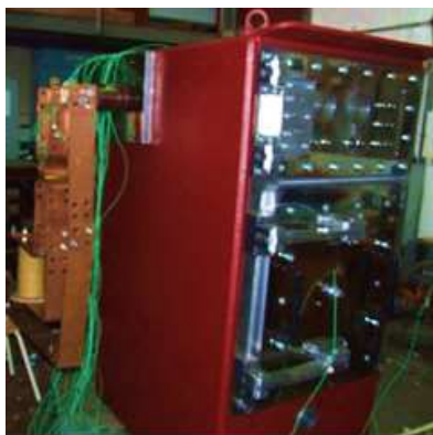
Fig. 1 View of distribution switchgear on the test stand
