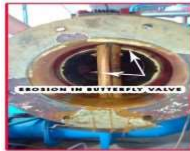
Fig.3: Erosion in Butterfly Valve
