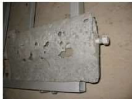
Fig.5: Erosion in the gate
