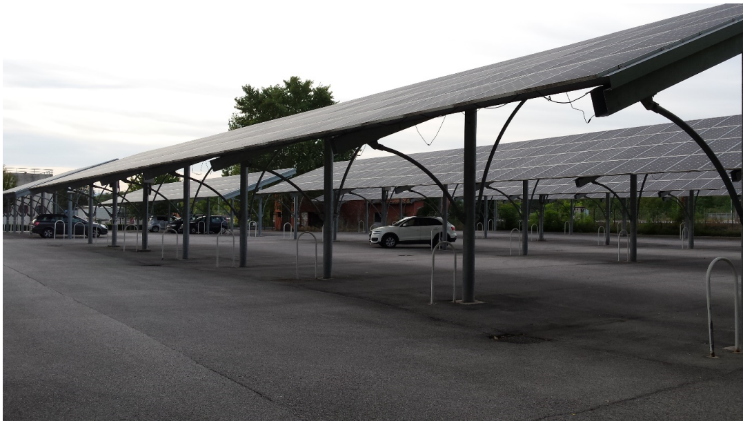
Figure 26: 185 kWp PV power plant at the Italian pilot site.
