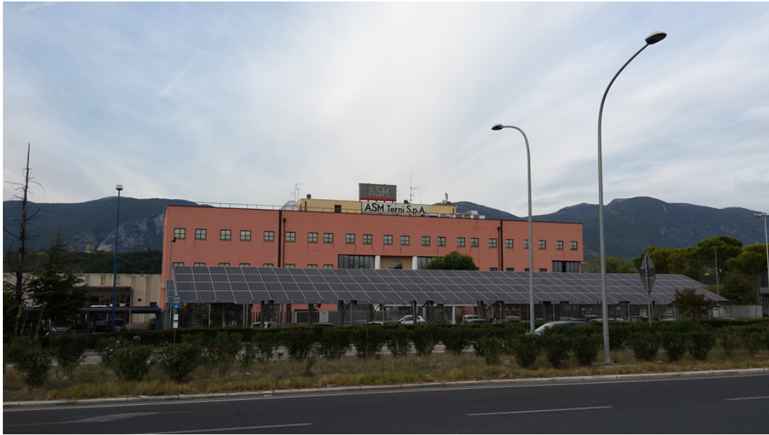
Figure 25: 60 kWp PV power plant at the Italian pilot site.
