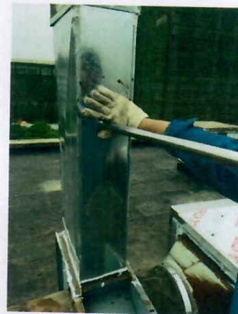
厨房油烟排气筒
