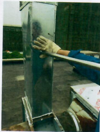
厨房油烟排气筒
