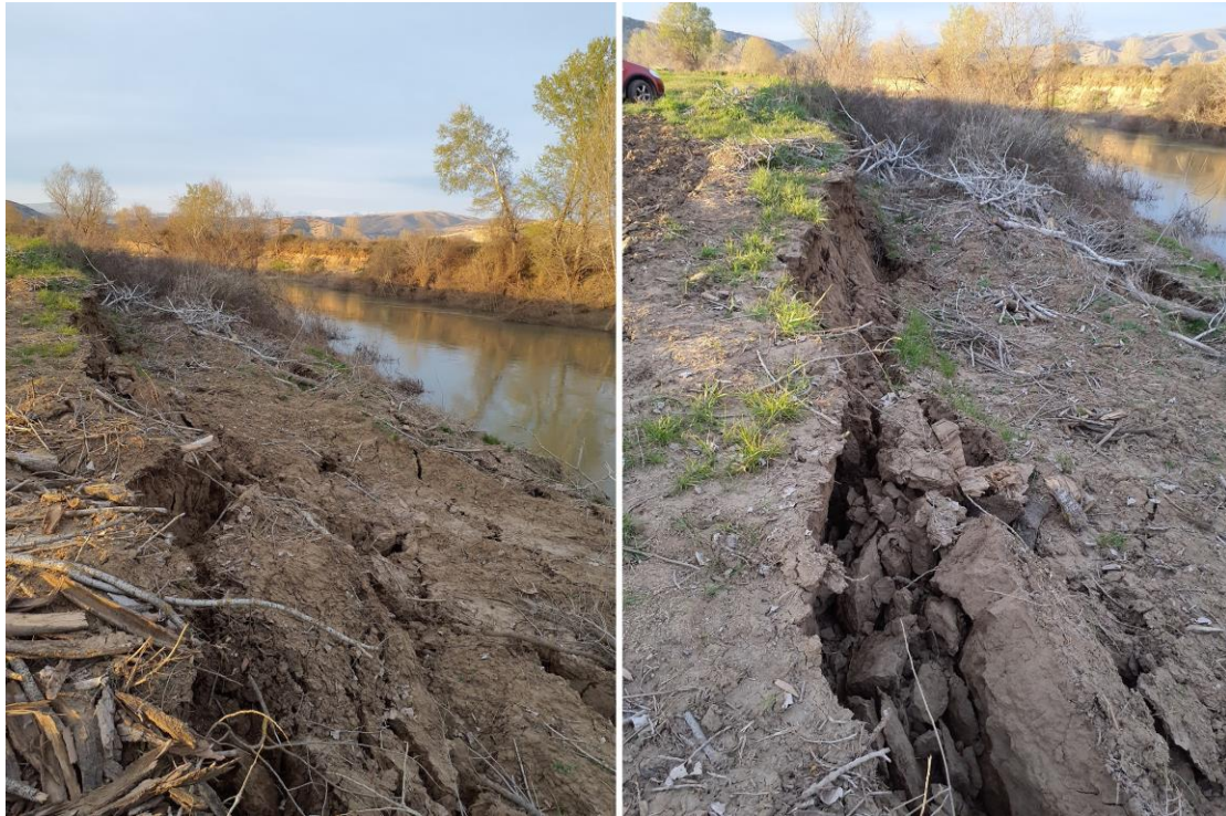
Figure 12. Lateral spreading along Pinios river (Photos taken by S. Valkaniotis 05/03/2021).
