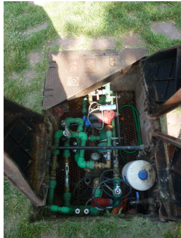
Figure 5: Experimental facility hydraulic system.
