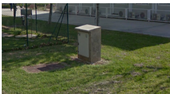
Figure 2: Location of borehole and control cabinet at UPV campus.
