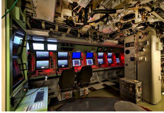
Figure 4: The Modified Control Room
