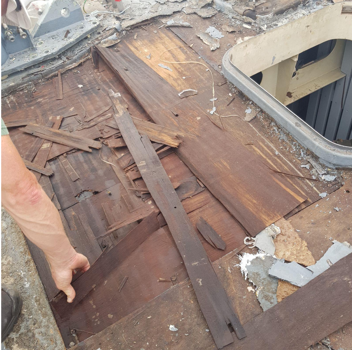
Figure 7. The layered nature of the Deck construction masked the extent of the water damage
