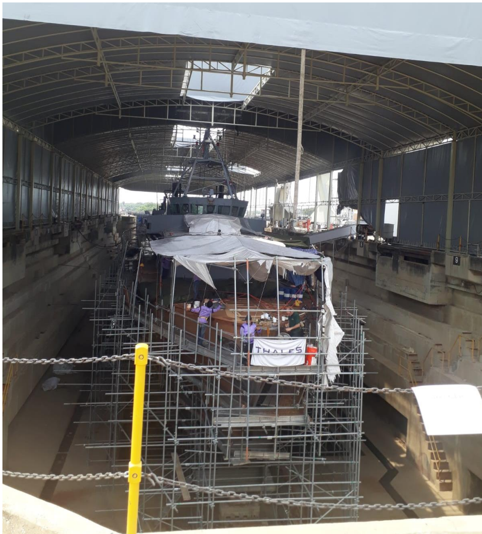
Figure 4. A tent was built over the open dry dock to protect the wood repairs from the elements
