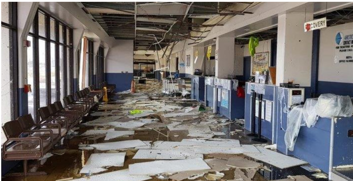
Destruction inside the Francisco C. Ada Saipan International Airport after Typhoon Yutu passed over the island. Photo by FEMA, 2018, courtesy of CNMI Office of Planning and Development.
