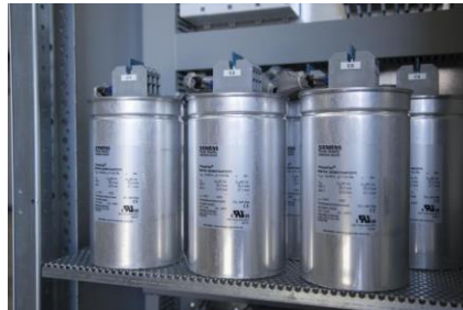
Figure 10 - Example of a capacitors bank
