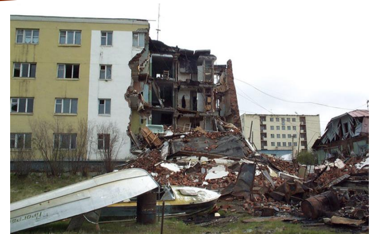
Thawing permafrost threatens buildings
