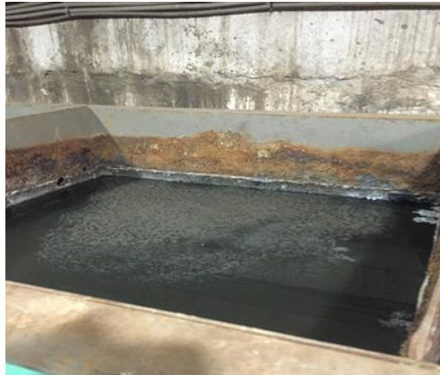
j. Comfort Home Estate wastewater sedimentation tank
