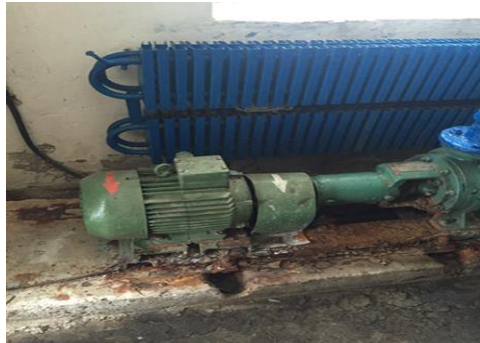
l. Old pump from WWTP
