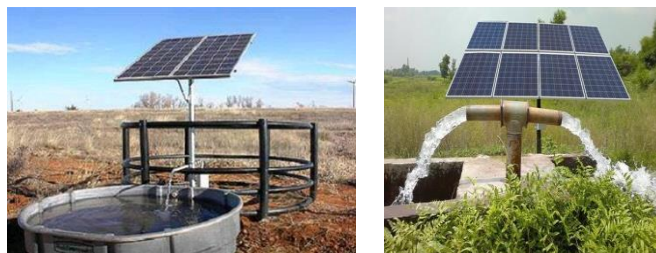
Figure 25. Solar water tank using motor
