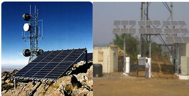
Figure 17. Solar operating mobile tower
