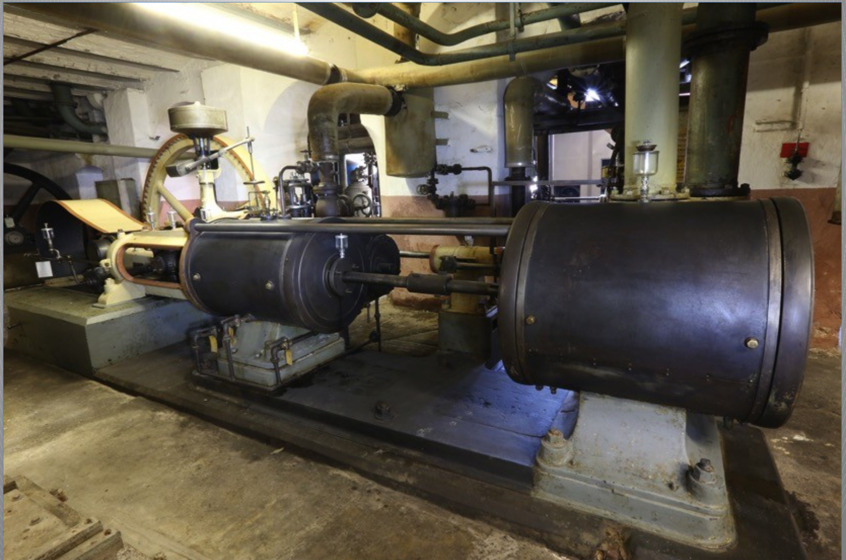
Extremely elongated horizontal one-cylinder steam engine with slidecontrol (1918): one piston rod for the steam and pump cylinders
