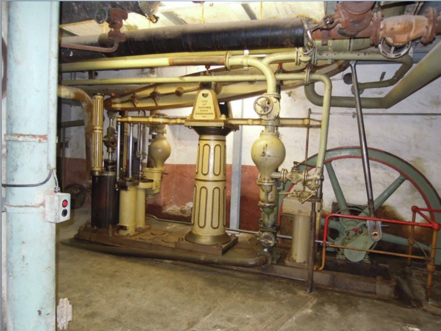
Beam steam engine built 1882 by Maschinenfabrik Sangerhausen, with a 2.700 mm diameter flywheel turning at 25-30 r.p.m., driving the lime milk pump (Reaktiviert)
