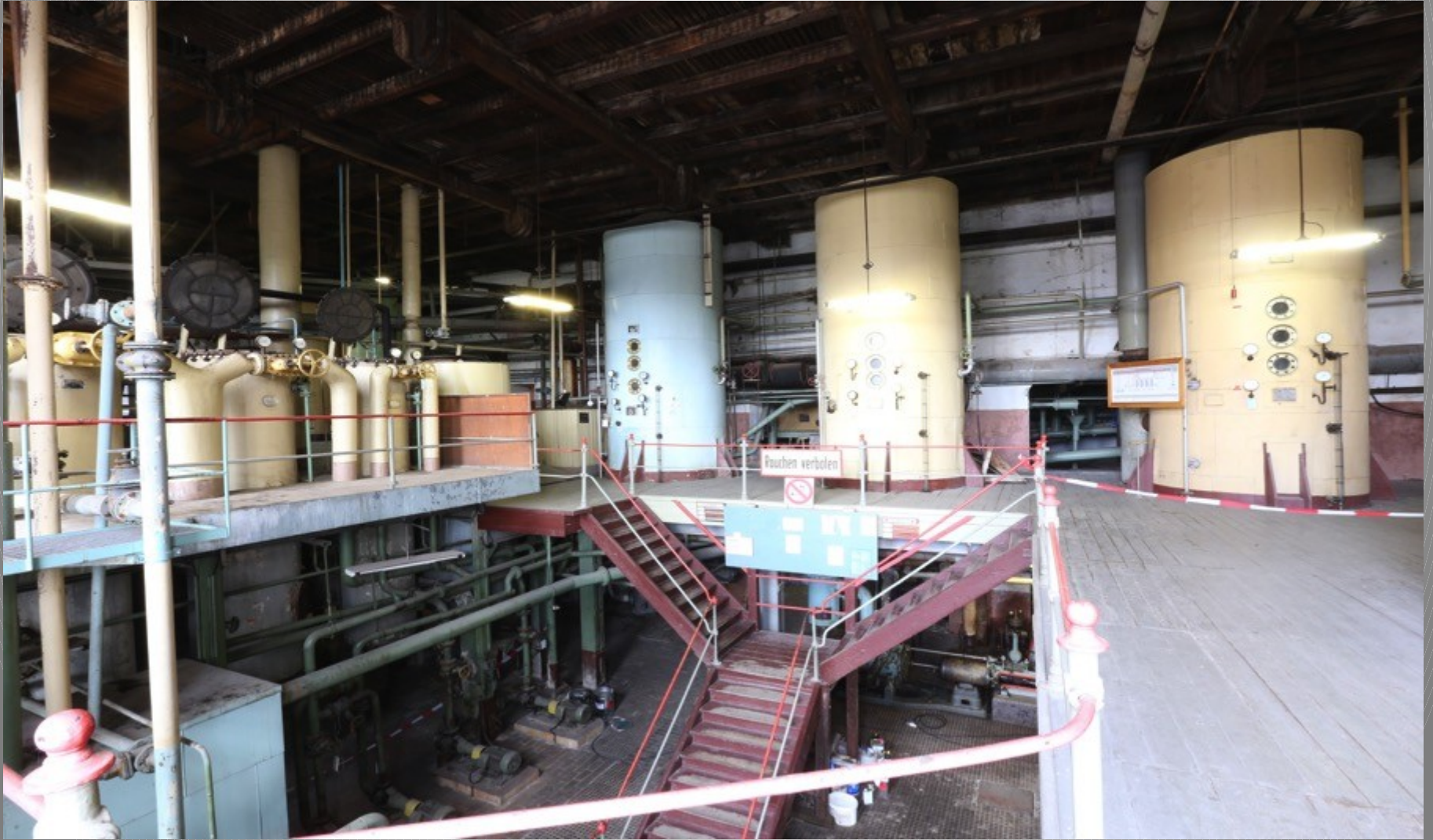
Staircase in the main building, the „Y“ configuration of wich is typical of beet sugar factories built in the last century
