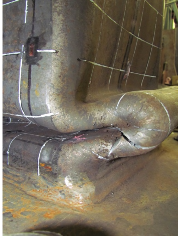
(f) North west corner fracture
