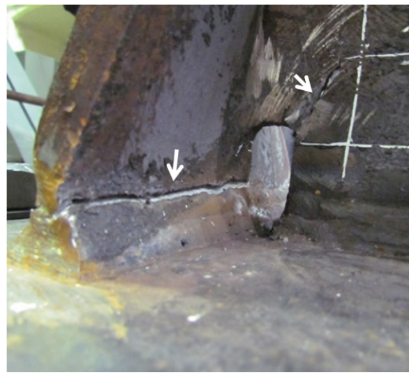
(b) flange weld toe and weld access hole (W-6-34-C2-V)
