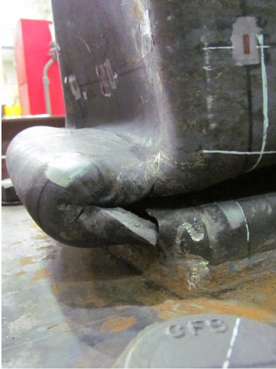
(e) North east corner fracture
