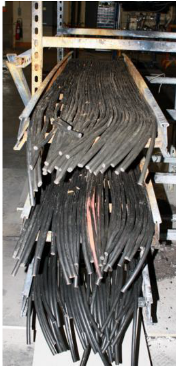
Figure 3. Photograph of the cable arrangement in MT3, taken from the CHRISTIFIRE report [15].
