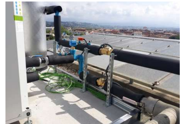
Control - hydraulic installation
