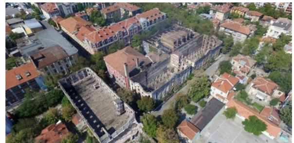
Fig. 9 The aftermath of the fire [16]
