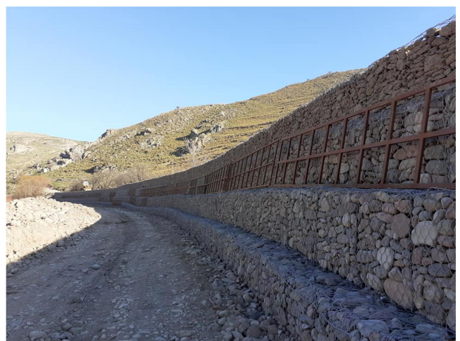
Photo showing the construction "Serazaneti" to stabilize the river bank and to enhance its capacity to accept higher stream power during the flood event (Taken by facebook page "Ο χρούσος")
