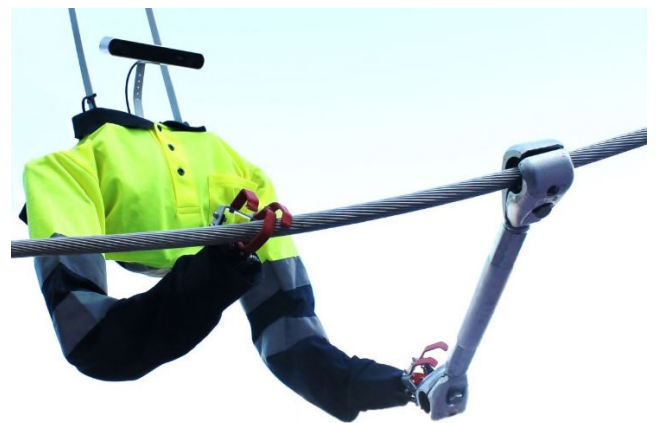
FIGURE 3. Anthropomorphic dual arm manipulator in long reach configuration installing a separator device on a power line.
