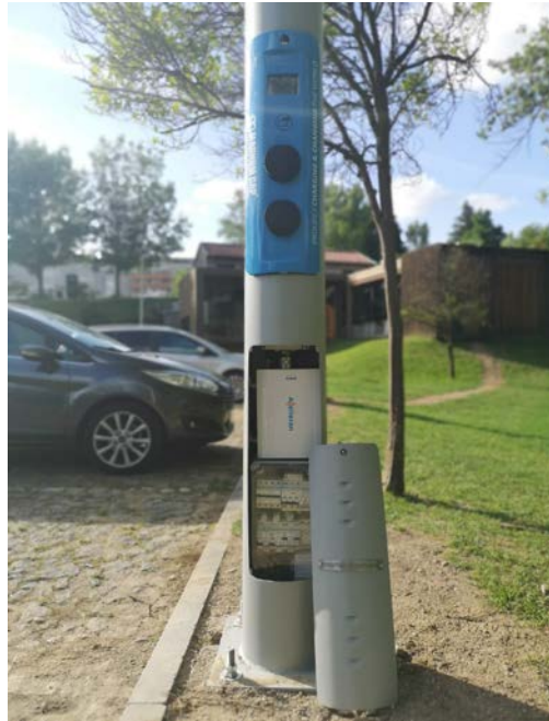
Figure 14 - Smart Lamppost (EV Charging & Telco modules)
