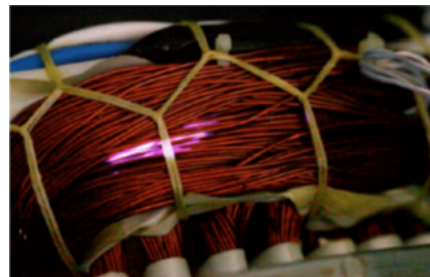
Fig. 1. A typical phase-to-phase insulation failure [4].
