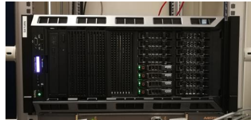
Figure 15: Edge Server 2 - SATURN.
