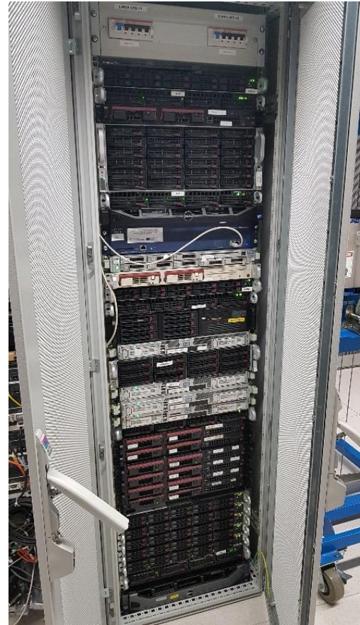
Figure 9: 5GCity Metro DC rack.
