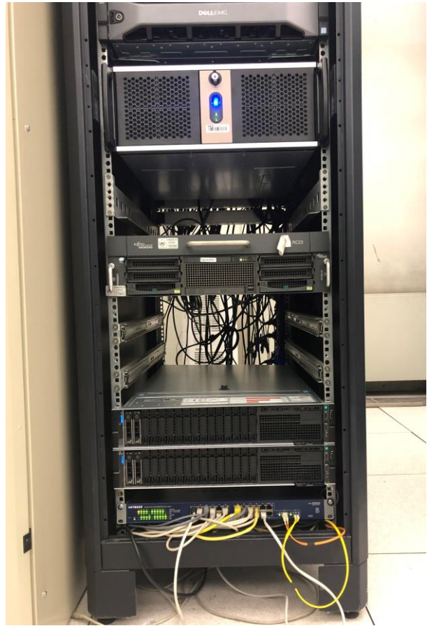
Figure 24: 5GCity Edge/Metro Node (VSP-DC). From the bottom of the rack: L2 switch; NFVI Servers (x2); UC1 Video Analytics Server.
