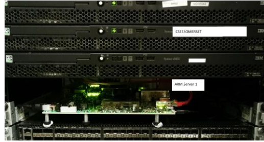
Figure 14: 5GCity Edge Servers at WTC-DC.
