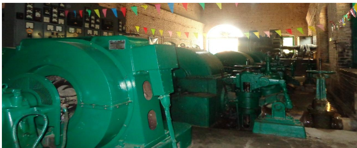
Fig.4:-Turbine at power house of Pharping Hydropower
