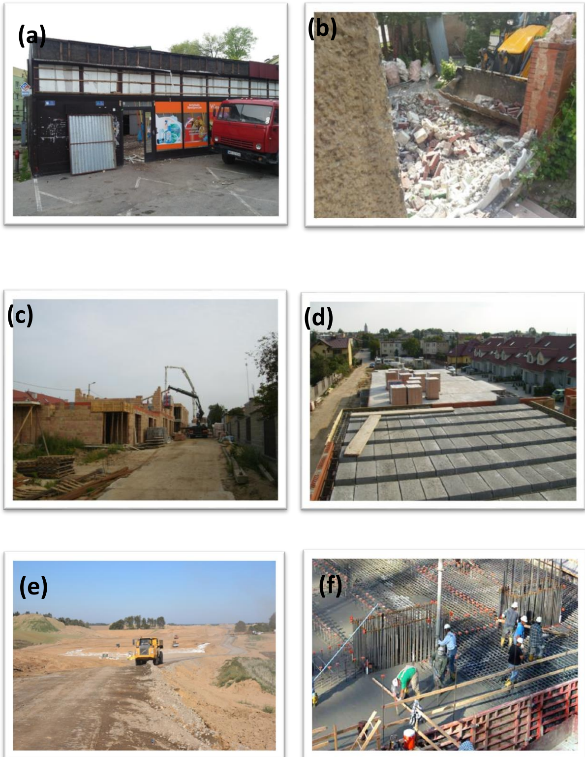
Figure 2 (a) Demolition - steel construction (b) Demolition – traditional construction (c) Construction works – new (d) Construction works – traditional (e) Construction work – roads (f) Construction work - Reinforced concrete technology
