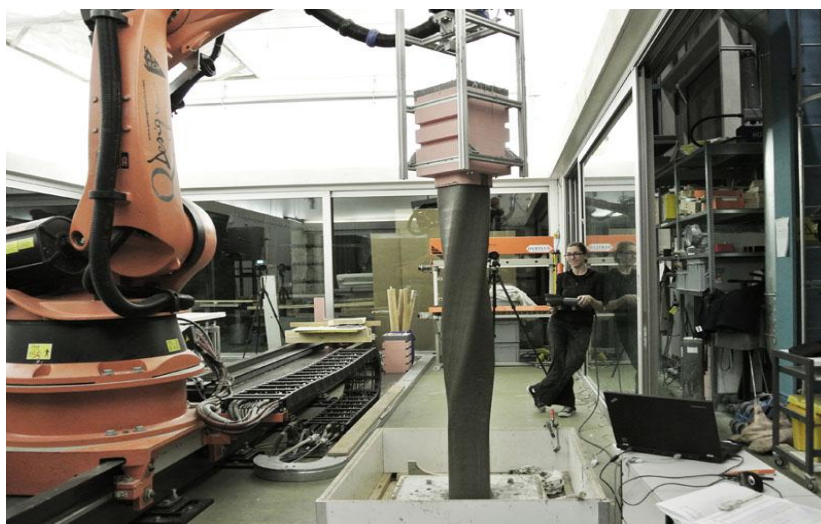
Fig.3:- Gramazio Kohler Research, ETH Zurich, Smart Dynamic Casting, 2013. (Source: http://gramaziokohler.arch.ethz.ch/web/includes/popup.php?projectId=223&Copyri ght=18&lang=e&BilderGezuegelt=1&image_count=4 , date accessed: 03 Dec, 2019)
