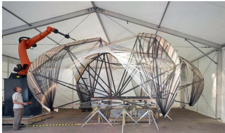
Fig.4:- Gramazio Kohler Research, ETH Zurich, The Programmed Wall , 2006. (Source: http://gramaziokohler.arch.ethz.ch/web/includes/popup.php?projectId=81&Copyright=18&lang=e&BilderGezuegelt=1&image_count=3&closeText=click%20to%20close , date accessed: 03 Dec, 2019)
