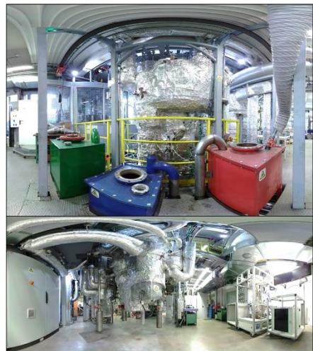
Fig. 2: Upper part and lower part of the DFB biomass gasification system
