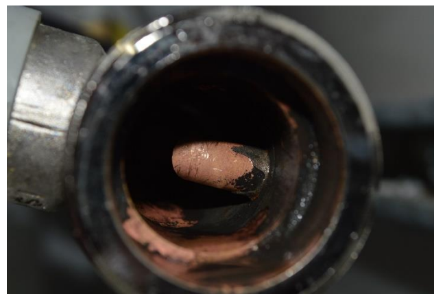
Fig. 1 Picture of a flow meter, where it is possible to observe depositions after two years of operation.
