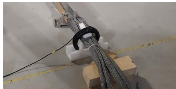
Figure 4: Rogowski coil installed in the ground side of the measurement circuit.
