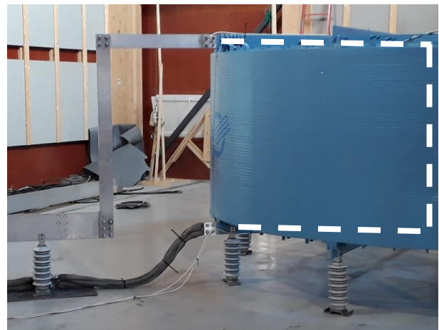
Figure 6: High voltage was connected to the upper terminal and ground return to the lower terminal. High-voltage measurement connection is shown as dashed white line.
