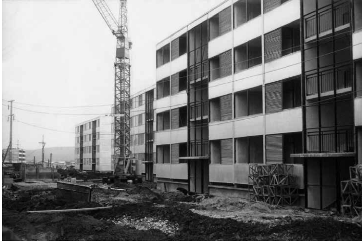
Prefab apartment buildings under construction. Source: Constantinos A. Doxiadis Archives. © Constantinos and Emma Doxiadis Foundation.
