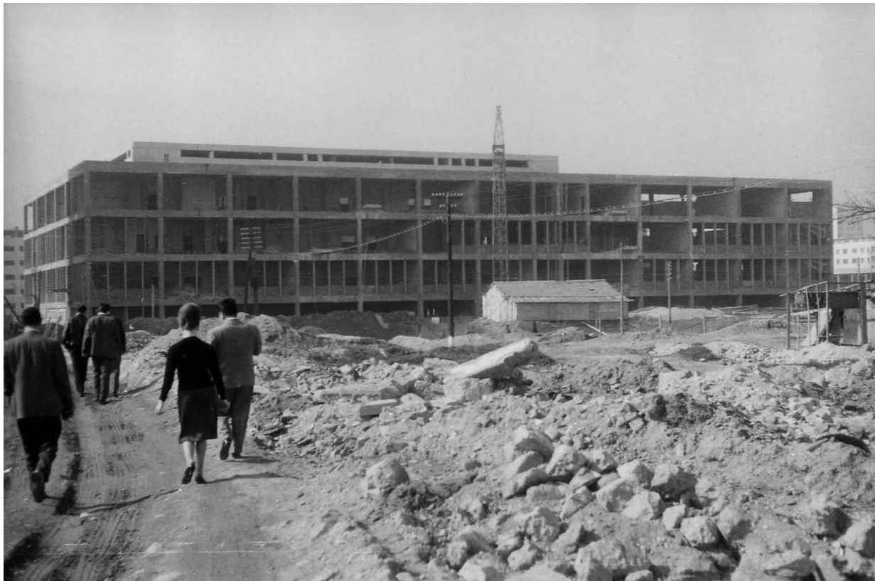
Faculty of Technology under construction and among the debris; its construction had begun before the earthquake. Source: Constantinos A. Doxiadis Archives. © Constantinos and Emma Doxiadis Foundation.
