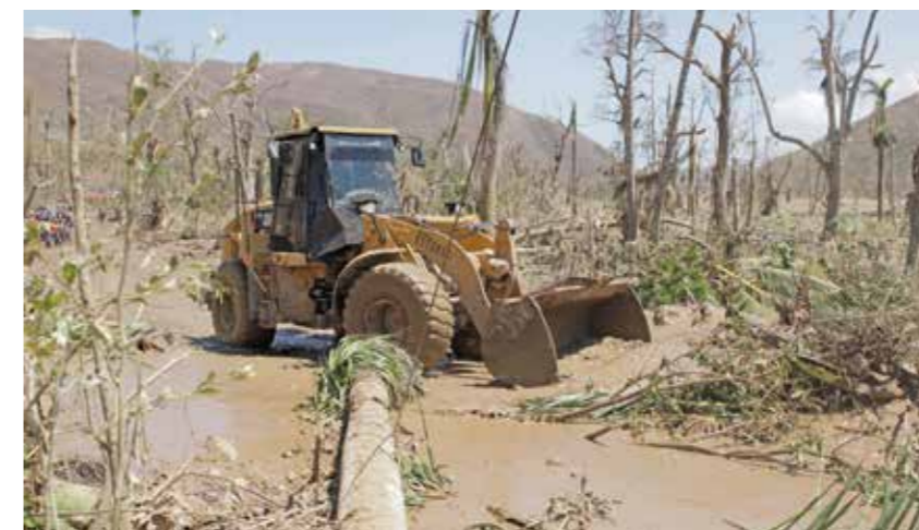
Figure 9.5 Haiti post hurricane Matthew 2016. © UNEP
