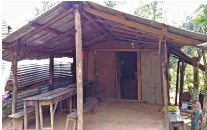
Figure 8.2 Vulnerable house in Nepal. © K. Sudmeier-Rieux
